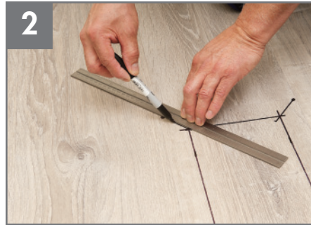
2 Mark diagonal stopping points on the four corners of the damaged plank.
