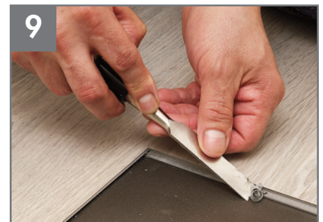
9 Remove the lock from the long and short edges of the surrounding material with a small chisel. Vacuum up debris.
