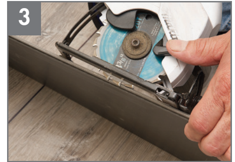
3 Use a plank as a gauge to set the saw blade to the proper depth to avoid cutting through the subfloor.
